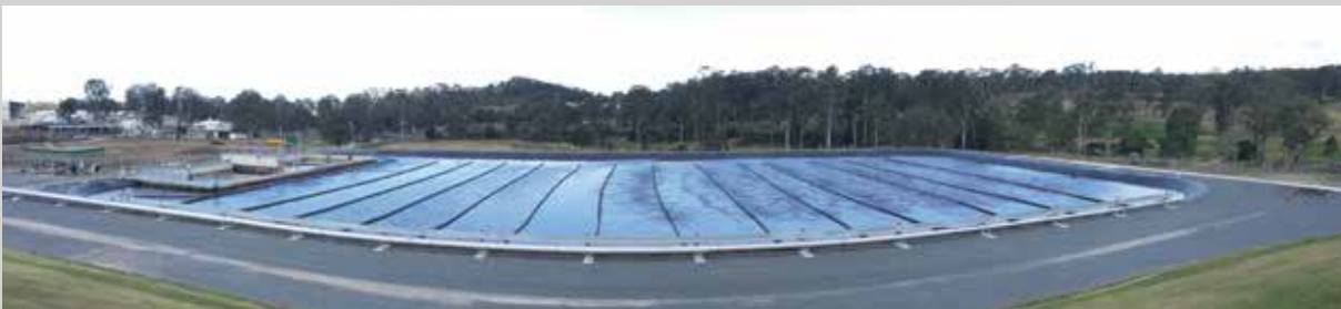
Teys Australia Beenleigh Biological Nutrient Removal (BNR) System
